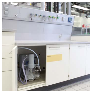
Laboratory with space-saving vacuum supply in the cabinet. Convenient pump control with integrated CVC 3000 E.
