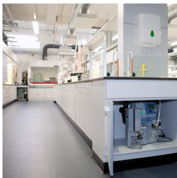
Vacuum network installation for the laboratory of a university, equipped with emission condenser Peltronic®, without additional cooling water connections inside the floor cupboard.
